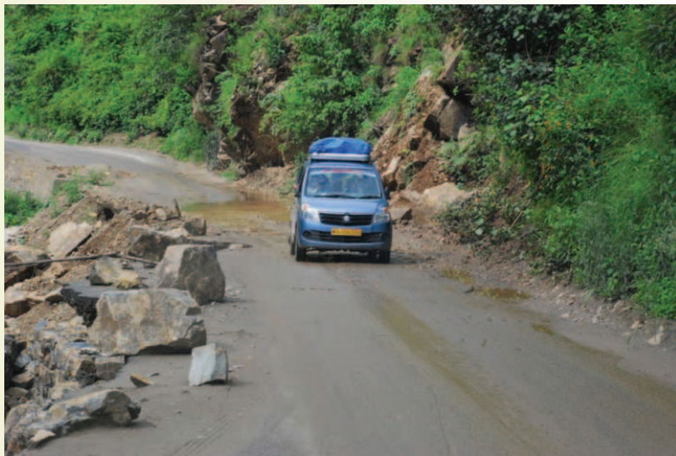
Road in Himalayas. Destruction of forests & landslide
