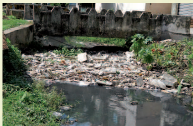
Waste plastics are littered around the drainage system causing health problems.
