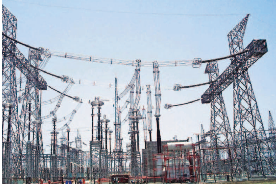
1200kV AC test station at BINA
