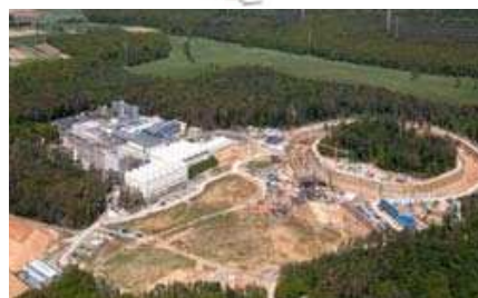
Facility for Anti proton and Ion Research (FAIR) under construction at GSI ( https://www.researchgate.net/figure/Facility-for-Anti-proton-and-Ion-Research-FAIR-under-construction-at-GSI_fig6_297368774 ; picture-alliance/dpa/GSI Helmholtzzentrum)
